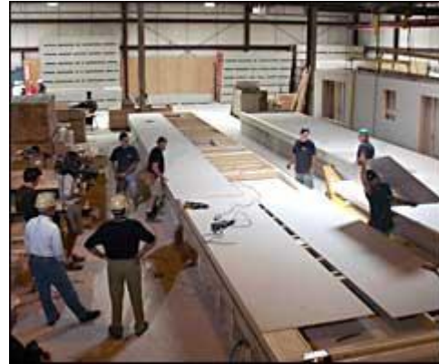
Weather-tight work conditions at the factory speed the modular home building process.
